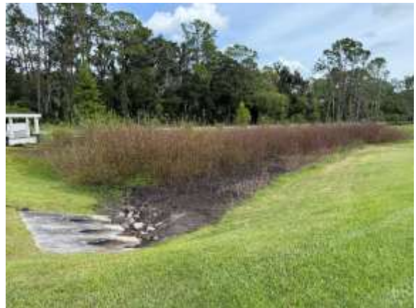
Wetland H (natural wetland area) No desirable species – needs clearing/replanting plan recommended
