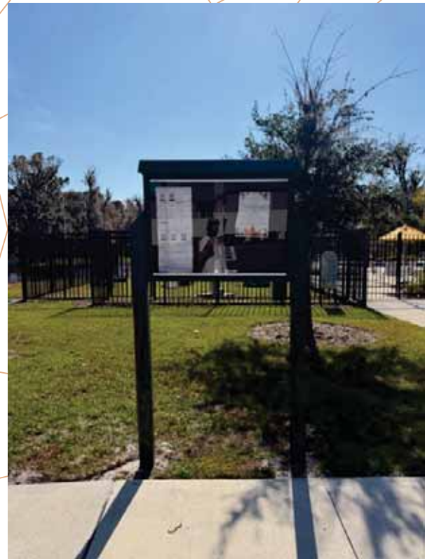
Message Board Install.
