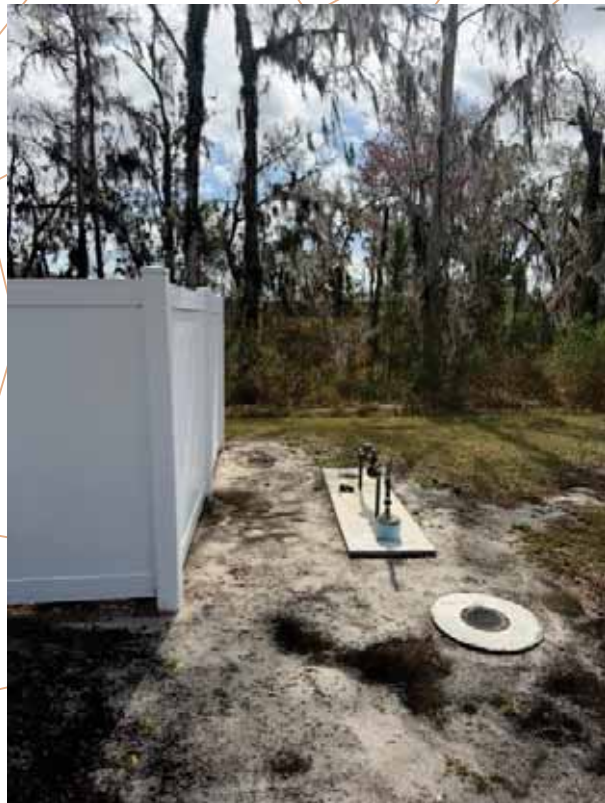
Pump Station near Pond 10
