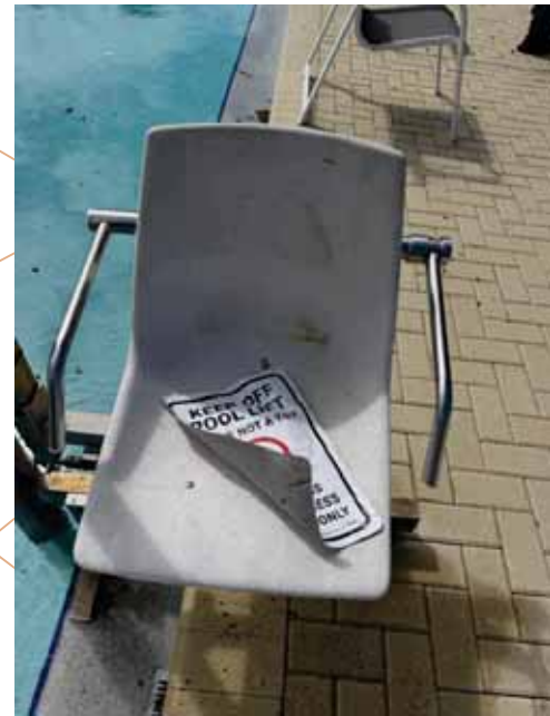
Handicap Chair Sign To Be Replaced.
