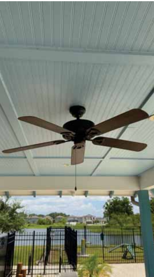
Outdoor fan that needs to be replaced.
